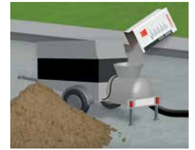
2 Adding the screed binder at the correct mix ratio to the aggregate
