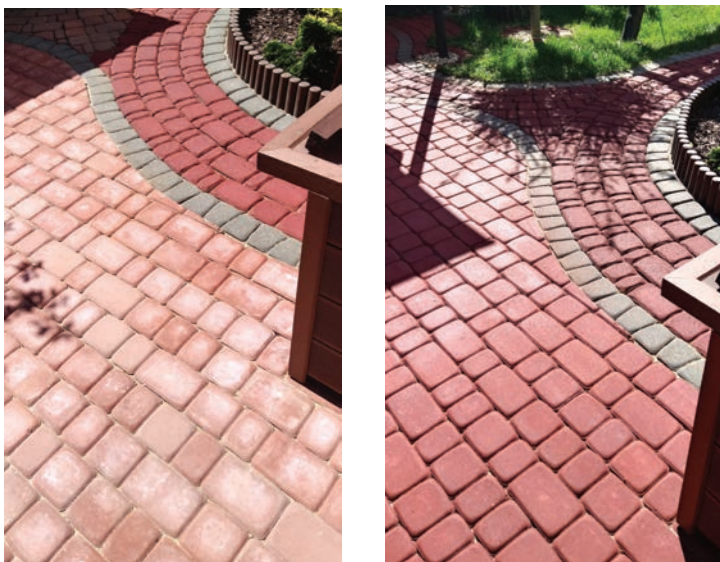
The effect of renovation works on concrete surfaces.
