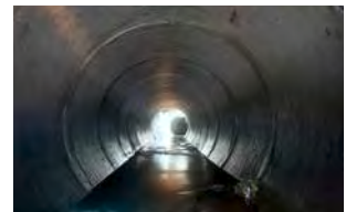
Sewage ducts and shafts
